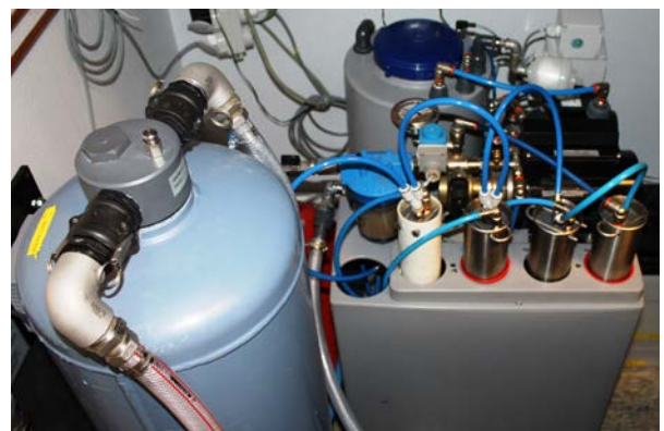
Fig. 2: The installed equipment used for cleaning printed circuit boards according to the Qlean-method at Flextronics in Karlskrona, Sweden.
